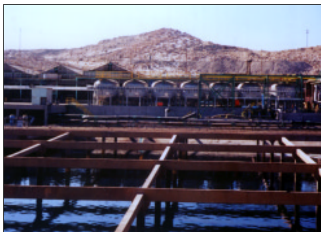
With systems in Peru, Chile, Mexico, Australia, Canada, and the United States, Smith & Loveless is the industry leader in SX electrolyte filter installations.
